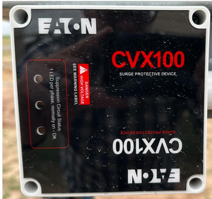
Figure 12 – Installed Well Pump Service Entrance Disconnect SPD
