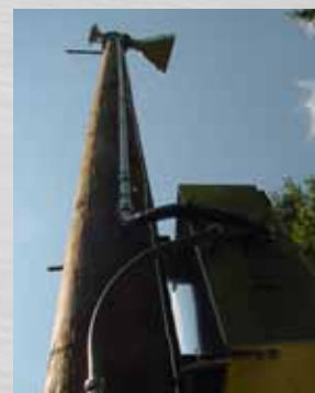
Mid-State Communications installation in Malta, NY
