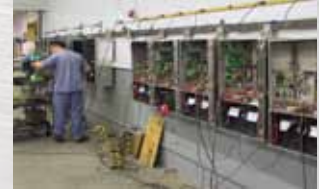
Testing Siren Cabinets
