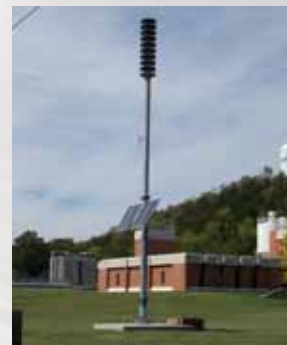
WPS2909 with solar panel
